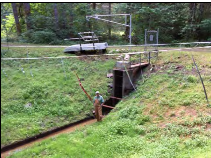
The water control structure is concrete on 3 sides with the fourth side designed to fit removable dam boards that control water depth. A culvert at the base of this structure runs below the earthen dam and out to Letz Creek.
