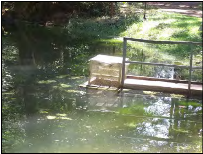
Top screened portion of the water control structure and pond outlet as seen at full pond stage.
